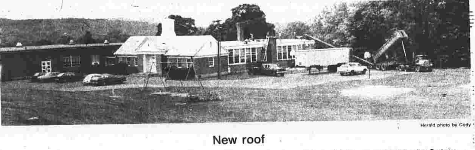
Workers last week began putting a new roof on the 1948 section of the Andover school building. Shown here laying stones, they are expected to complete the roof this week. It is being put on by Roofing Systems — Narotsky Inc. of West Haven for $10,535.
